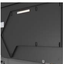
Inspection access panel for filter and heat recovery unit
